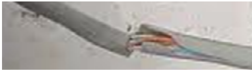
Damaged Non-UV Cable
